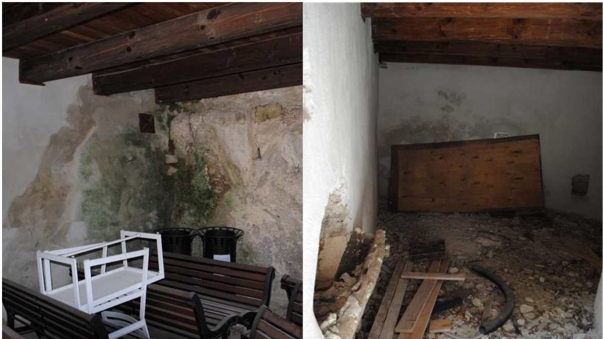
Figure 5. Degradation of the interior.
