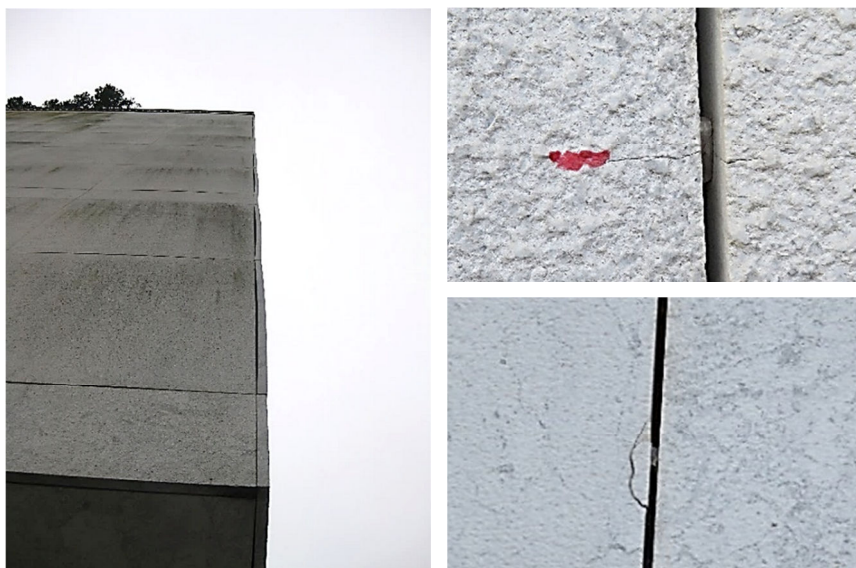
Fig. 4 - Examples of bowing and local damage/fracture detected on the marble slabs
