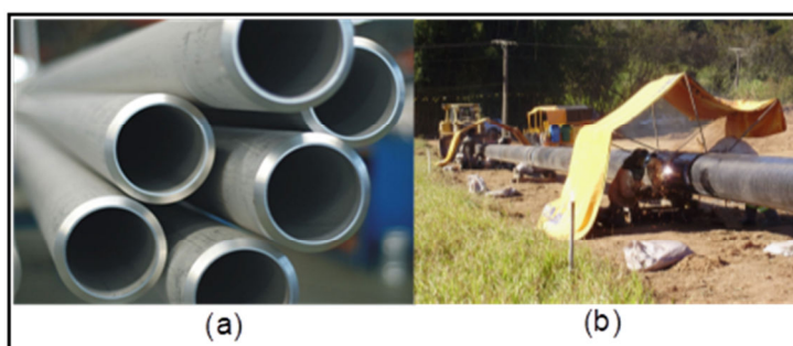
Fig. 1 - (a) Tubes prepared with machined bevels (source http://www.chilexpo.com/ consultation on 05/06/2017); (b) top welding of the tubes forming a column (Source: Petrobras collection, 2010)
