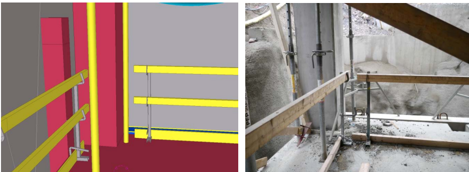
Figure 45. Comparing model and live situation: Safety railing detail in the corner of the slab.
