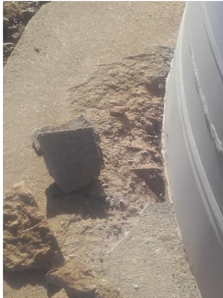
Figure 1. Concrete spalling at the interface between the steel tower and concrete pedestal.
